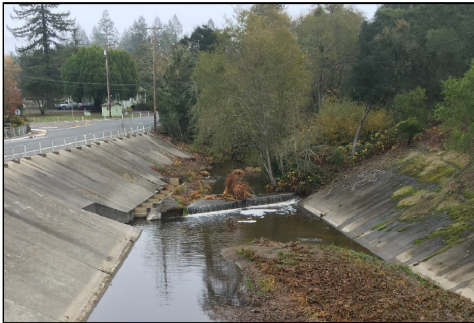
Figure 2.1-3: Photographs of Vortex Tube Rehabilitation Project Work Areas. Top: view of the downstream (north) side work area and outlet of Vortex Tube, foreground shows concrete embankment along Montgomery Drive. Bottom: view of the upstream (south) side work area at concrete weir and fish ladder that connect to the Vortex Tube.
